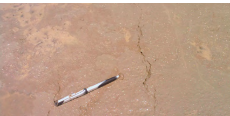
An example of concrete bleed and plastic shrinkage cracking.
