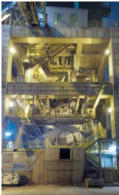
FCB Horomill® in Barroso plant (Holcim, Brazil).
