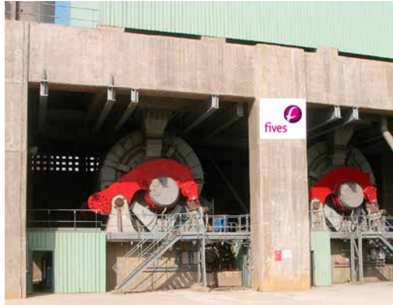
Twin-FCB Horomill® in Thai Nguen plant (Vinaincon, Vietnam).
