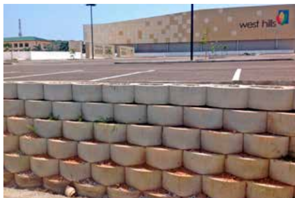
Retaining walls at West Hills Mall – a major shopping centre in Accra West.
