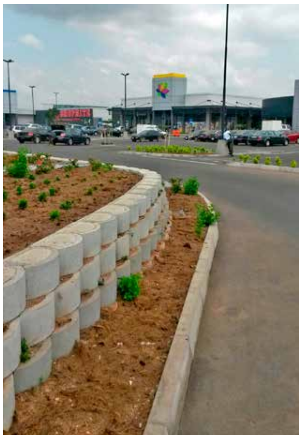
BessBlock's Terraforce retaining walls at Achimota Retail Centre, Atterbury Property's latest shopping mall development to be completed in Ghana.
