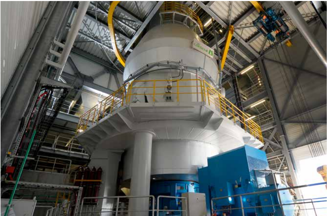
A Loesche cement mill like this LM 46.2+2 in Duisburg, Germany, was installed in the Nova Cimangola factory in Luanda.
