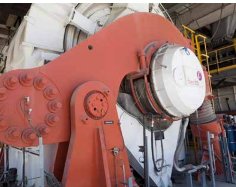
FCB Horomill® in Hermosillo plant (Holcim-Aspasco, Mexico).
