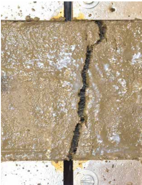
Figure 2: Direct tensile test on fresh concrete clearly showing the fibres bridging the crack even after extensive crack opening.
