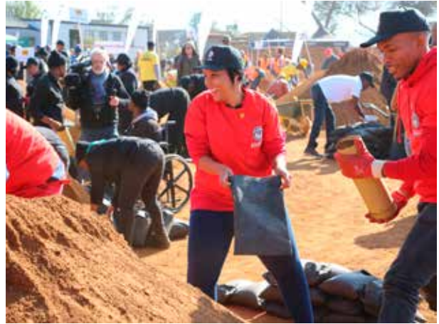
PPC staff members, including the executive team attempted to fill 1000 sand bags which will be used to fill the cavity walls of the Devland campus building
