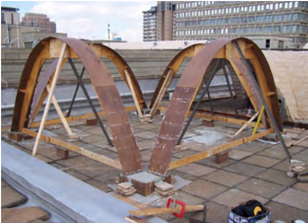
Placement of catenary guides.
