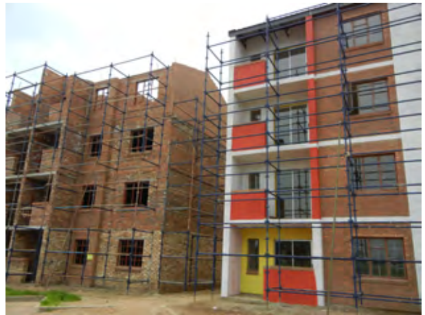
Two blocks at City Deep Green, Johannesburg, being built by the Motheo Construction Group using Elematic hollow-core slabs.
