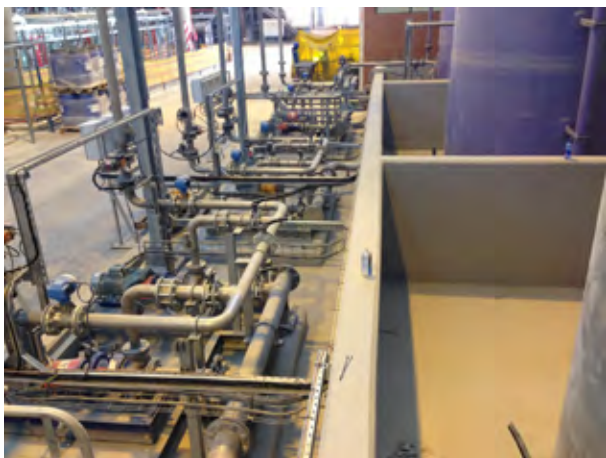
Nyeleti Consulting Engineers specified numerous specialist Sika products for repairs and protection of various areas of the plant.
