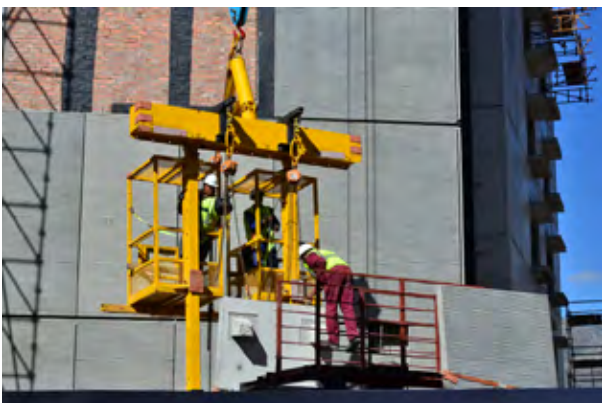
Workers attach chains to a textured concrete panel prior to lifting by a specially manufactured crane. The protruding corbels can be clearly seen on the panel's inner face.
