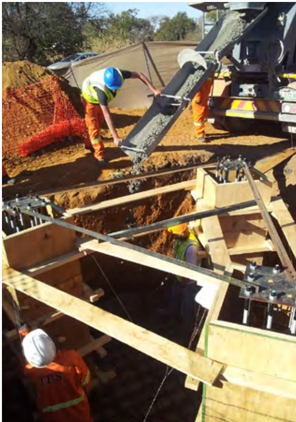
Readymix can be placed exactly where it is needed and eliminates the need for site mixing.
