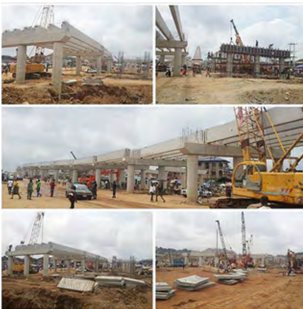
Construction of 6-Lane flyover bridges at Sapon and Itoku to feed 10-lane Boulevard from Lafenwa to Sapon, Abeokuta.
