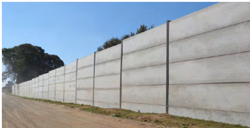
Sections of recently completed prestressed hollow-core slab walling at the Echo Prestress factory in Chloorkop.
