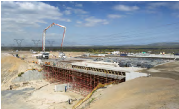
Civil infrastructure projects, such as the N7 Melkbos and Atlantis Interchange in the Western Cape, require specialist concrete products with superior handling and placing characteristics.
