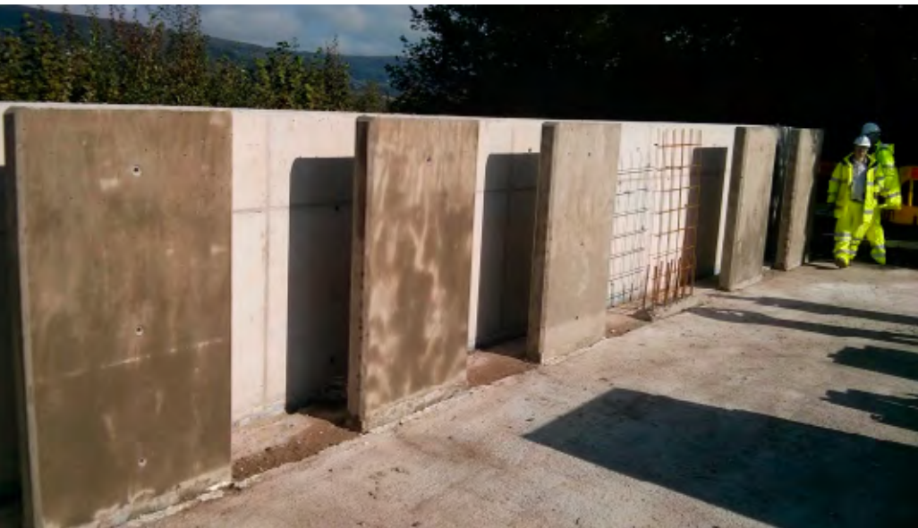
The Materials for Life project is piloting the real-world tests of three self-healing concrete technologies. Led by Cardiff University School of Engineering, M4L is supported by Costain and other industrial partners. Photo: Cardiff University UK.
