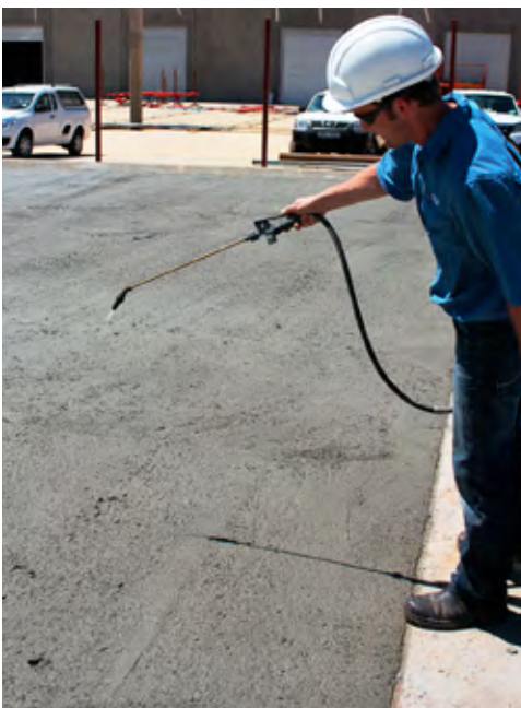
The duration and type of curing applied during the setting process will play a determinant role in enabling the concrete to achieve the strength and durability that is required to meet the design parameters of the structure.
