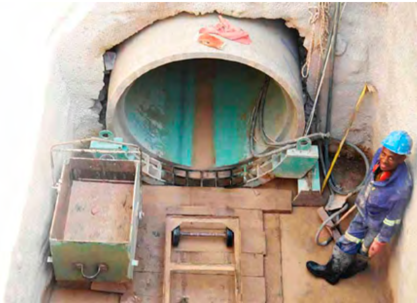
The 148,840 m of jacked Rocla pipeline required the manual excavation of 370 m 3 of rock.
