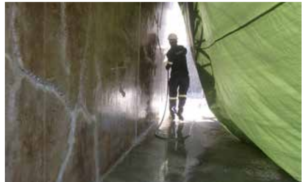
Sanika's crack repair at Impala Platinum slag granulation cooling tower in Rustenburg.
