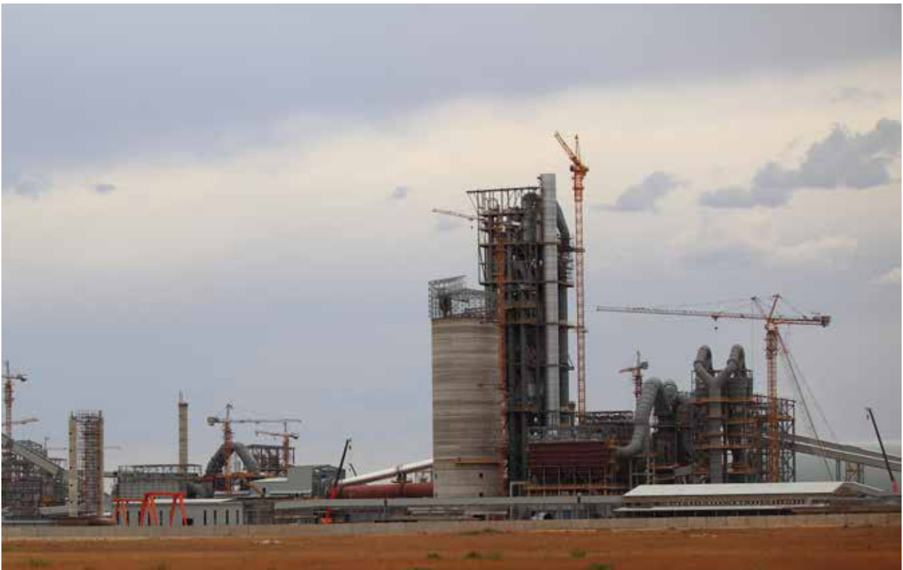
Sephaku Aganang plant uses the latest and most high-tech equipment.
