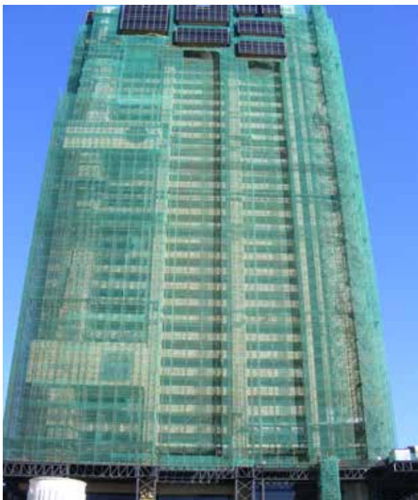
ABSA Towers during application of polyurea and drilling for anchoring new façades.
