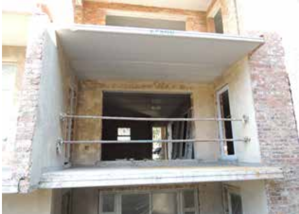
Projecting, cantilevered boxes formed with ESA slabs add interest to The Epic apartments.
