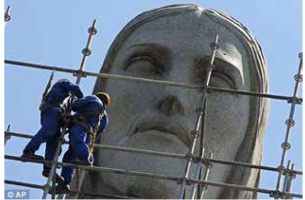
It takes scaffolding - and nerves of steel - to repair this iconic statue.
