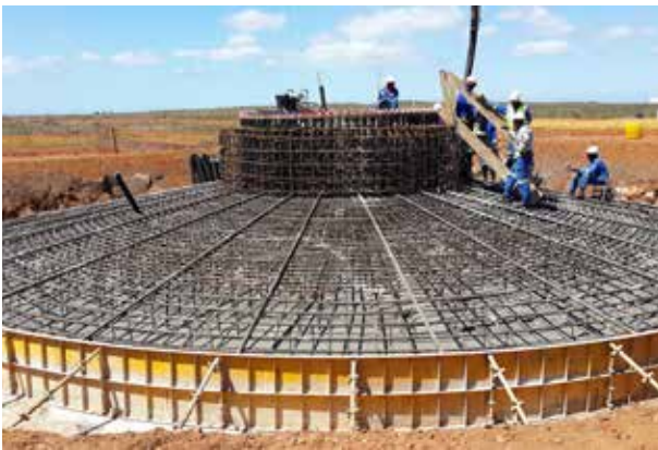
Each of the turbine foundations at the Jeffreys Bay Wind Farm project required approximately 335 m 3 of concrete and AfriSam was selected as the supplier of choice for this project.
