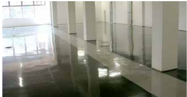
a.b.e. Construction Chemicals' abeflo system was used for new flooring at the Land Rover premises in Hillcrest, Durban.
