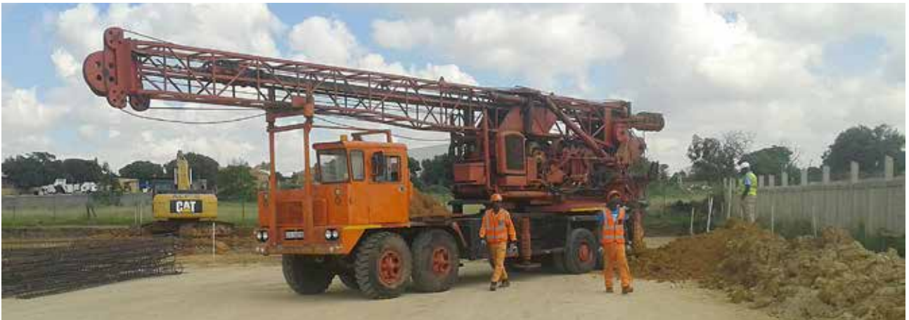
Gauteng Piling is using two auger rigs for the Value Logistics warehouse project: an MF and LDH machine. The rigs provide exceptionally high drilling speed which allows sufficient time to place the concrete and also helps to remove the risk of collapse and ingress of water inside the bore.
