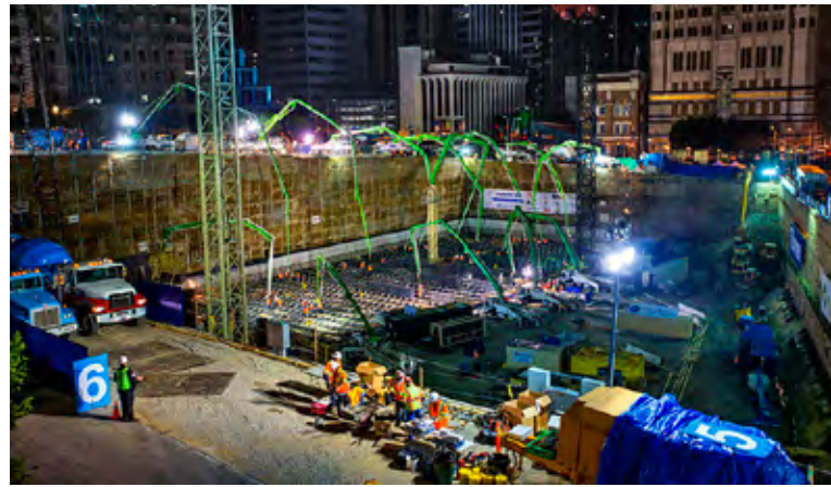
Turner construction set a new record for the longest continuous concrete pour for the Wilshire Grand Center in Los Angeles - 18.5 hours.
