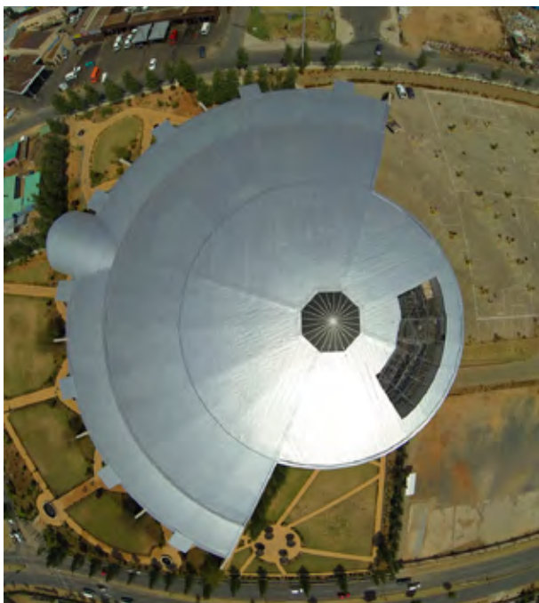
Multi-Dex 2000 used Mapei's Polypaint Alu when refurbishing the dome-shaped roof of the UCKG church in Orlando West.
