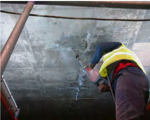
Sanika Waterproofing specialists recently used Kryton Krystol Technology to waterproof the Turbine Hall's basement car park.
