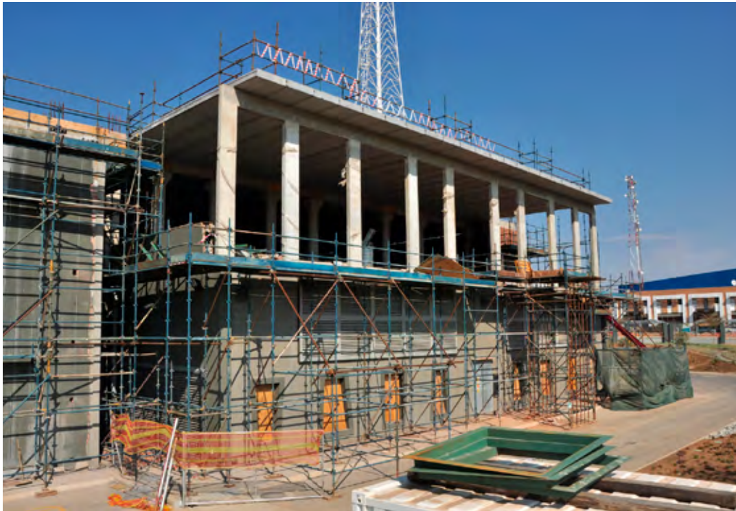
Phase 2 of MTN's Centurion data centre takes shape using Echo prestressed slabs.
