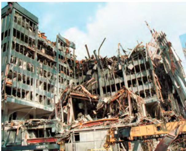
An example of concrete infrastructure in America not being repaired or sustained.
