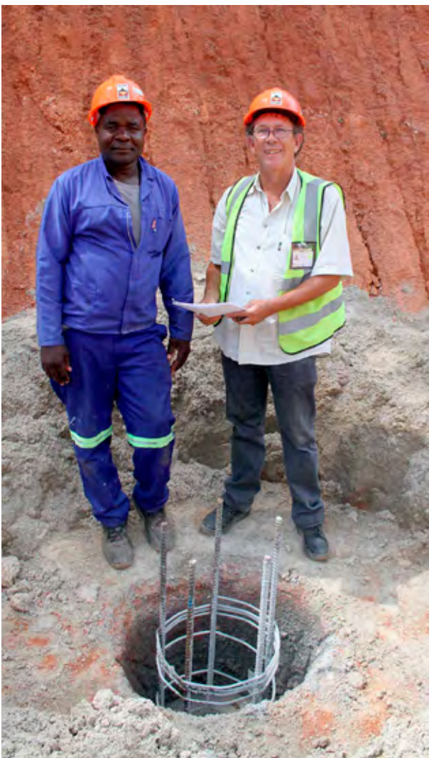
Gauteng Piling site manager, Kobus Geyer (right) and the site foreman, Alfred Phiri, in discussion at one of the completed piles for the Houghton office block.
