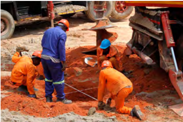
Gauteng Piling site staff performing a checking operation to ensure that the rig's flight is drilling at precisely the correct underground point. A thin peg is then placed in position at the bottom of the pile to guide the flight point to the exact drilling point to ensure optimum vertical boring.
