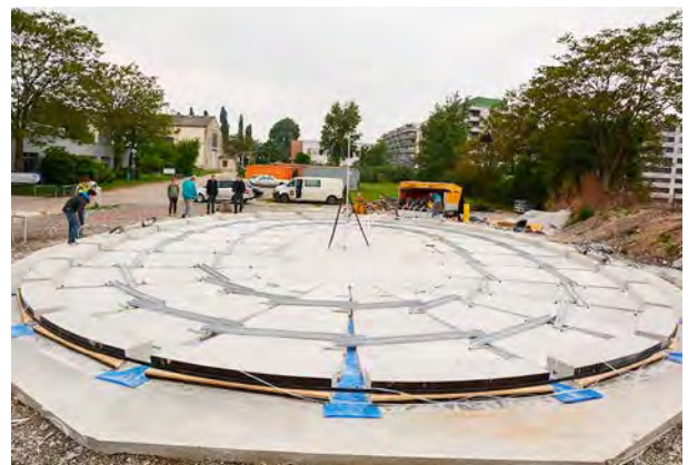
The dome-shaped cushion is inflated, lifting and bending the slabs. The cable is tightened to bring slabs together.
