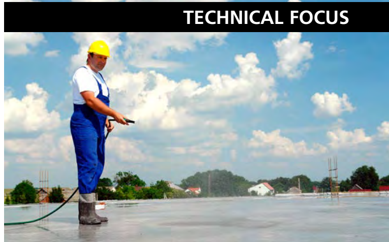
Don't allow concrete to dry out during the curing process, The Concrete Institute has advised.
