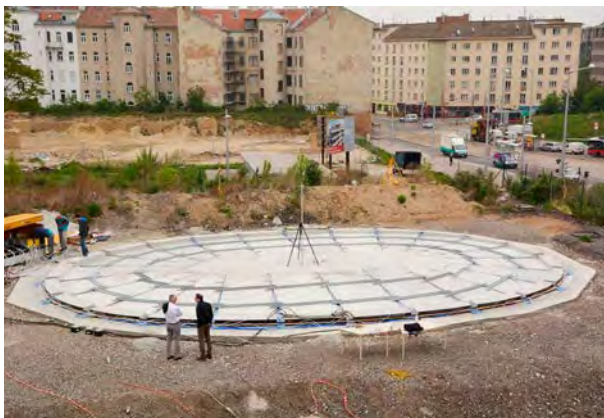
Concrete is poured into the forms and allowed to set, creating a series of flat slabs.
