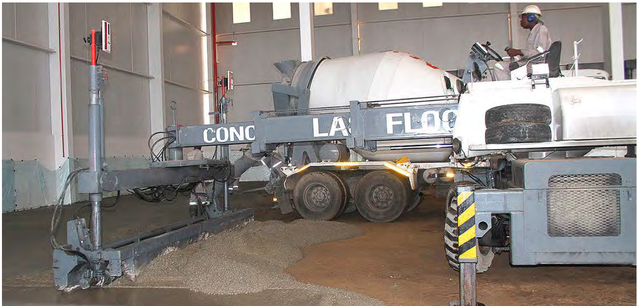
CLF's new Titan Top dry shake spreader machine in action providing strong, abrasion- and slip-resistant flooring for a new warehouse in Boksburg.
