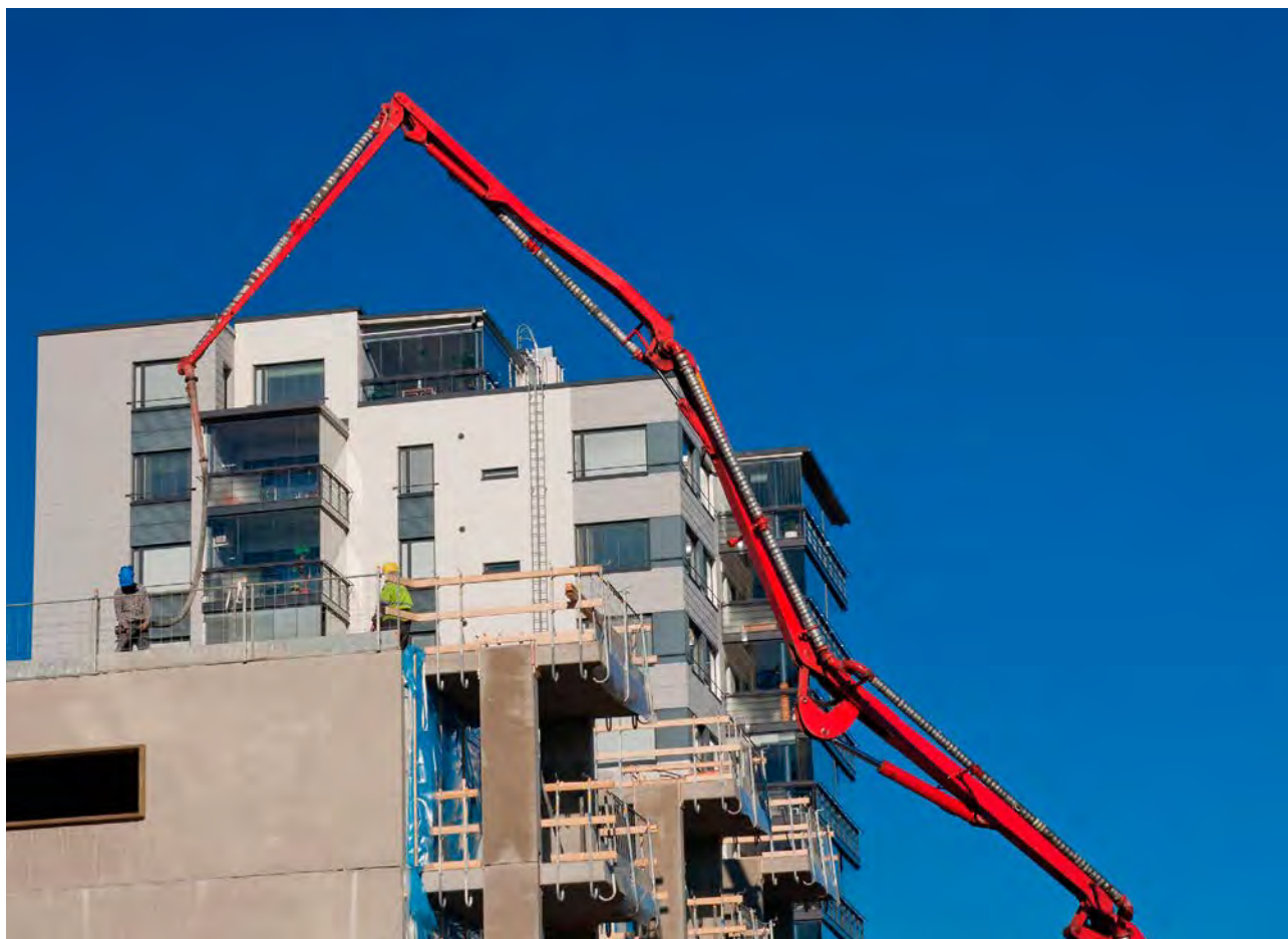
It is vital to look at the concrete pumping application and determine the most appropriate admixture that will fulfil the requirement.
