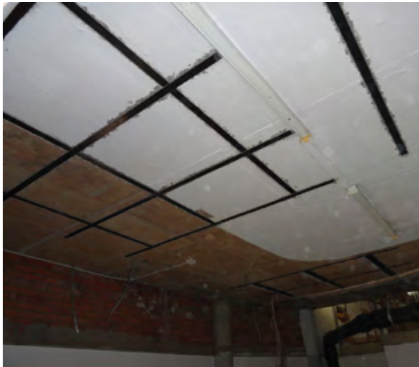
Sika CarboDur plates are installed onto the ceiling to strengthen the concrete slabs.
