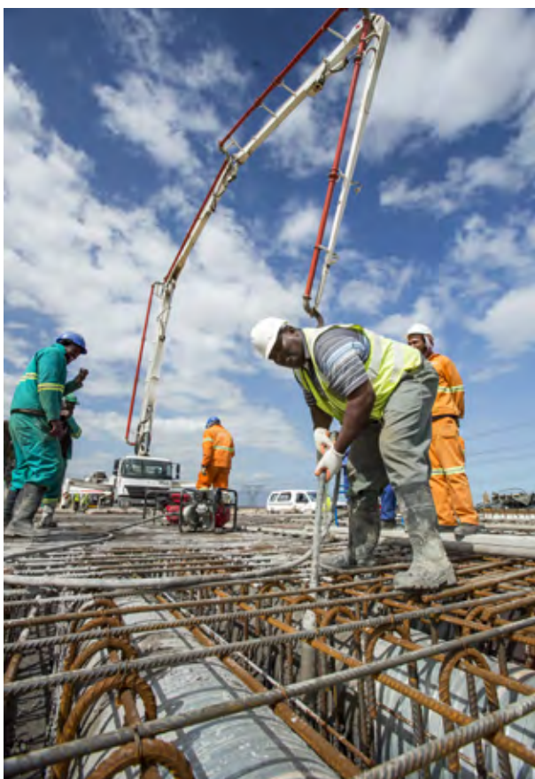
Prior to commencement of the project, AfriSam worked alongside Haw & Inglis to develop durable readymix designs that complied with the specifications for the interchange bridges.
