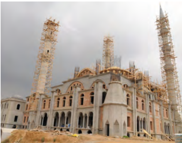
The structure begins to take shape with 600 craftsmen brought from Turkey working on its construction.
