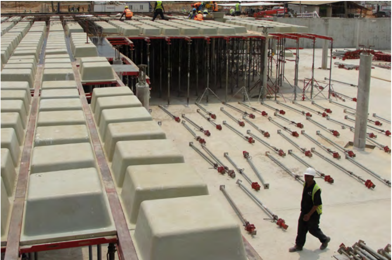
West Hills Mall in Accra, Ghana. Coffers on the Kwik-Deck system supported on BS props.
