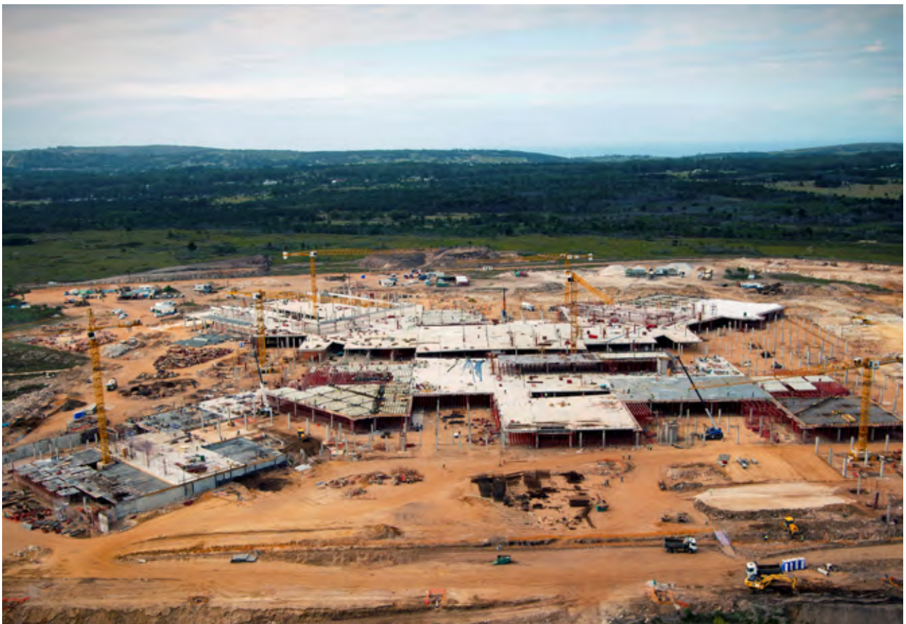
Baywest Mall in Port Elizabeth. Just one of the many malls under construction using Form-Scaff's Kwik-Deck system with coffers.
