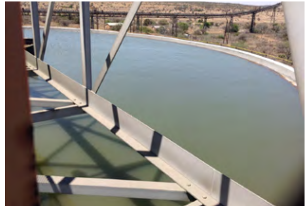
Anglo American conventional thickener waterproofed from the exterior using Kryton Krytol Waterproofing methods.
