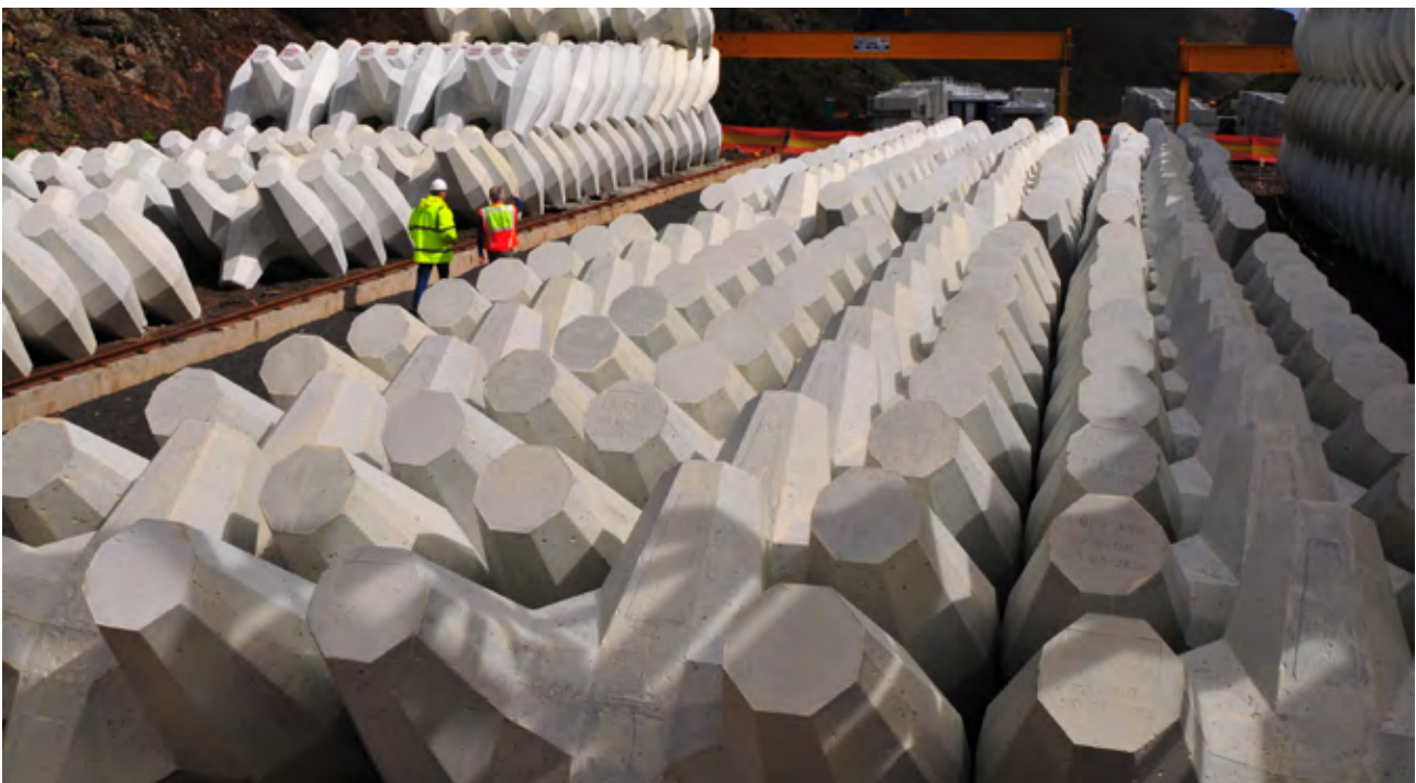
Over 700 units of precast Core-loc armour units (7 tonnes per unit) and hollow blocks (27 tonnes per unit before being filled with stone) were placed by crawler cranes via GPS around the wharf from the surface bed to just above sea level.
