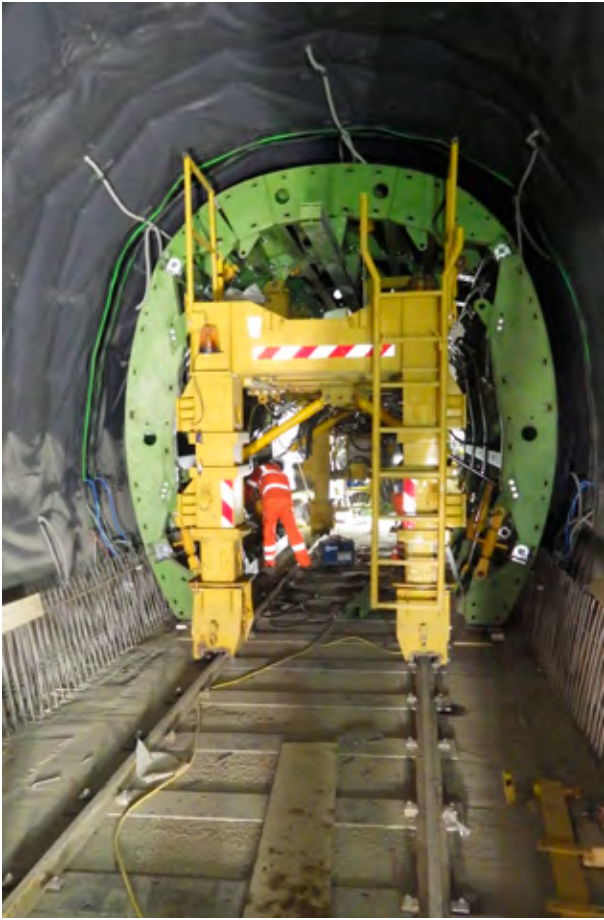
PAL22 with shutter installed.
