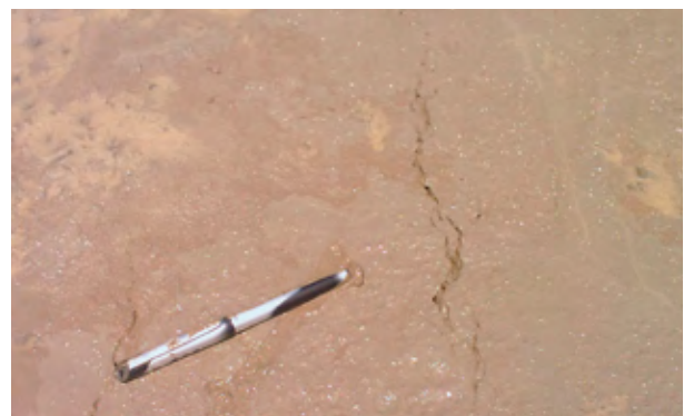
An example of concrete bleed and plastic shrinkage cracking.
