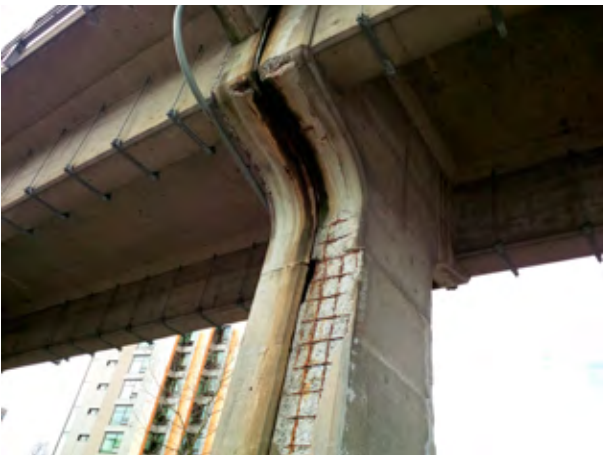
Corrosion initiated by cracks in the concrete provides paths for water and salts to reach the reinforcement. Corrosion is quite severe despite thick concrete cover to steel (up to 75 mm). This shows how significantly cracking can compromise the structure.
