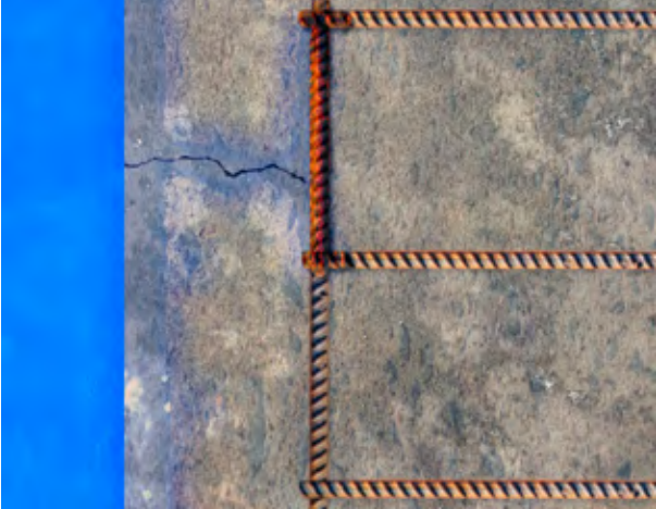
Corrosion will occur if there is moisture and oxygen present at the surface of the unprotected steel.
