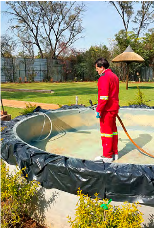
Noel Abendroth, head of a.b.e.'s Polyurea Performance Coatings Division, applying VIP Polyurea Quickseal LP65 waterproofing to the water feature at Number 7 on Brae Conference Centre in Pretoria.
