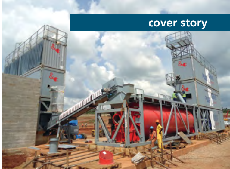
Above and below left: Kampala Cement's Plug&Grind plant.
