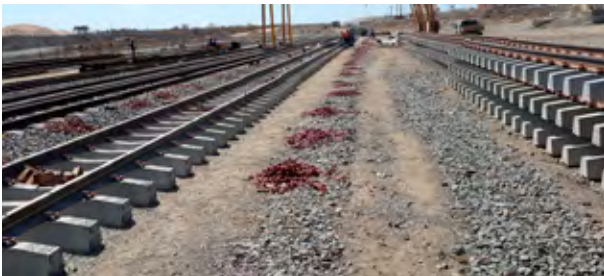
abe - railway sleepers Tete to Ncala line': Chryso SA supplied the admixtures and demoulding oil for the production of concrete railway sleepers for Mozambique's Tete to Ncala railway line.
