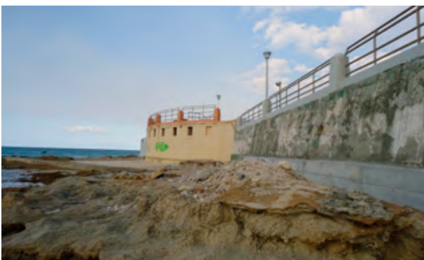
Before Sika repairs.
