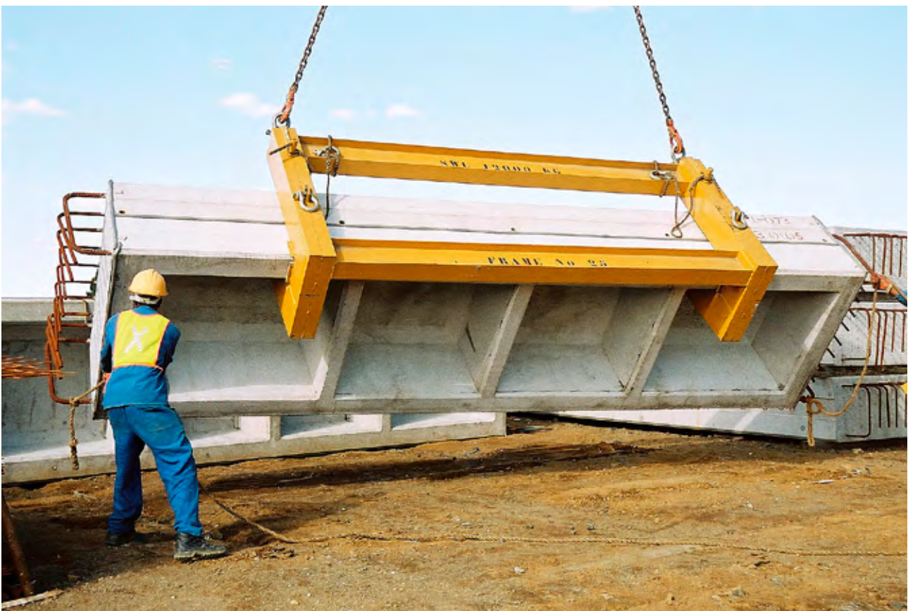
Precast concrete elements can be transported to a construction site and then lifted into place.
