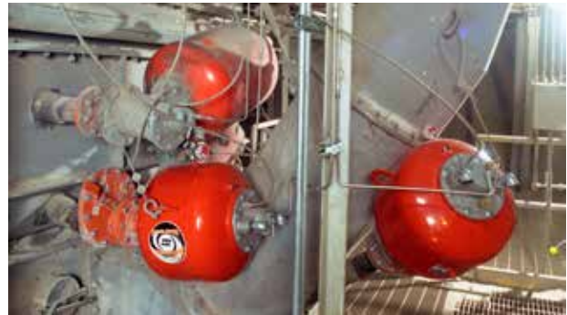
110 Martin® Hurricane Air Cannons are installed in the two plants, covering preheater towers, additive silos and cyclones.
