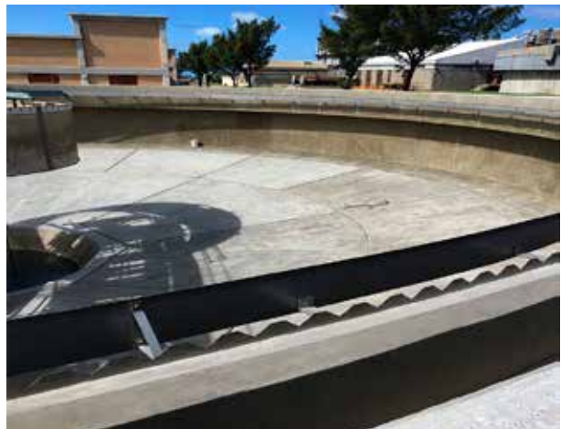
Clarifiers - repaired with monotop spall repairs with 612, walls skimmed with 720 epocem, all joints done with pro 3icure, surfaces treated with 903+ and 705L.
