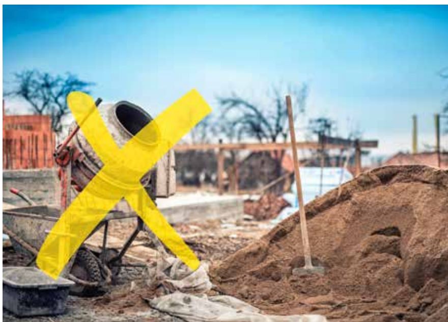
With the half cubic metre of material delivered to site ready to use, unsightly construction sites are a thing of the past.
