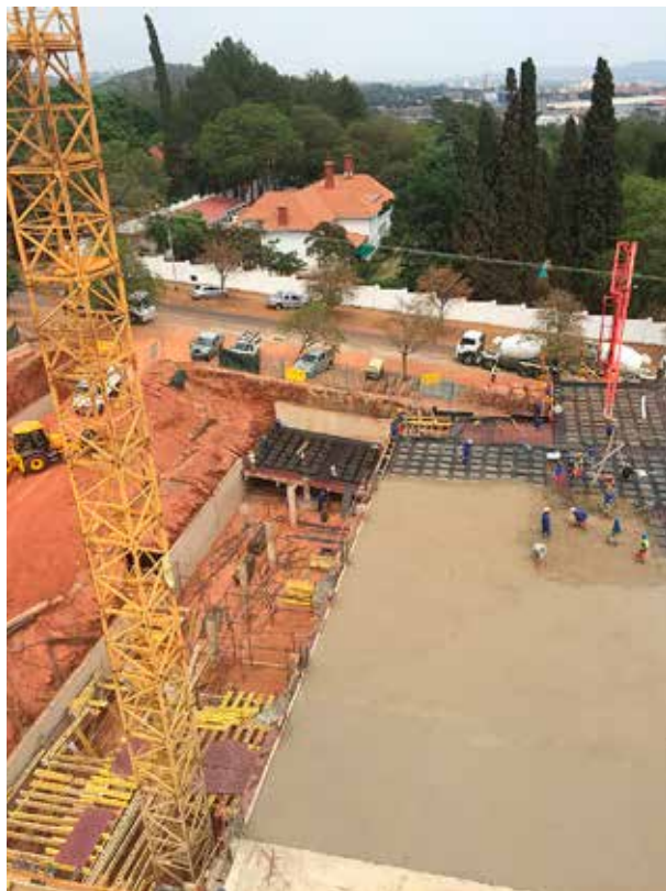
CHRYSO Macro Fibres were used for all the surface beds for the basement and parking areas at the ZA Hospital's consulting rooms being constructed by Mike Buyskes Construction.
