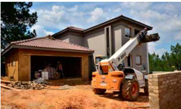
One of six new duplex cluster homes at the Brandi-Ann residential estate in Roodepoort being built by Renico Construction using Echo Floors reinforced hollow-core slabs for the upper floor sections.
