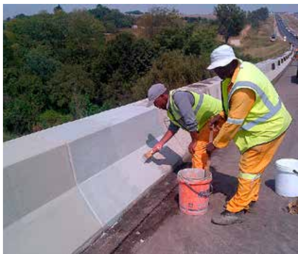
Work in progress on the N14 highway bridges for which a.b.e. Construction Chemicals is supplying three products.
