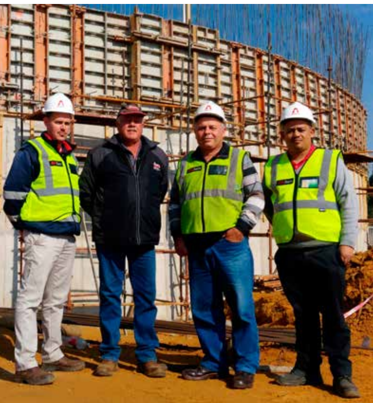
The 20-megalitre Droogheuwel bulk water reservoir underway in Randfontein; with the first concrete pour conducted in April, the structure is scheduled for completion in March 2018.
