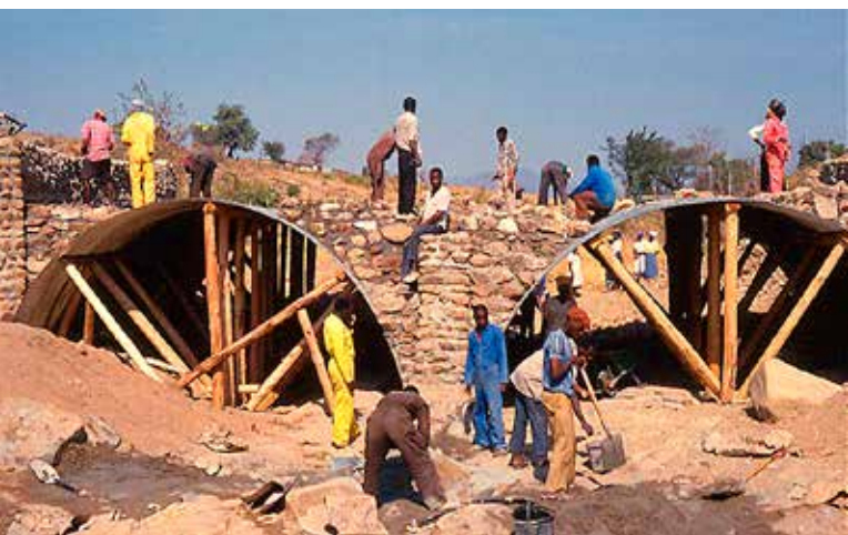
Construction of Rubble Masonry Concrete dams and bridges is very labour intensive. (Photo: Dr. Rod Rankine).
