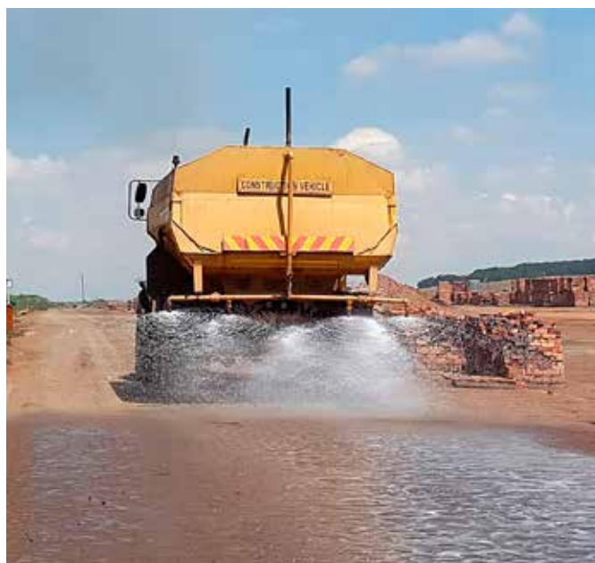
Chryso Eco Dust is easy to apply to road surfaces with a water tanker fitted with a liquid distribution bar.
